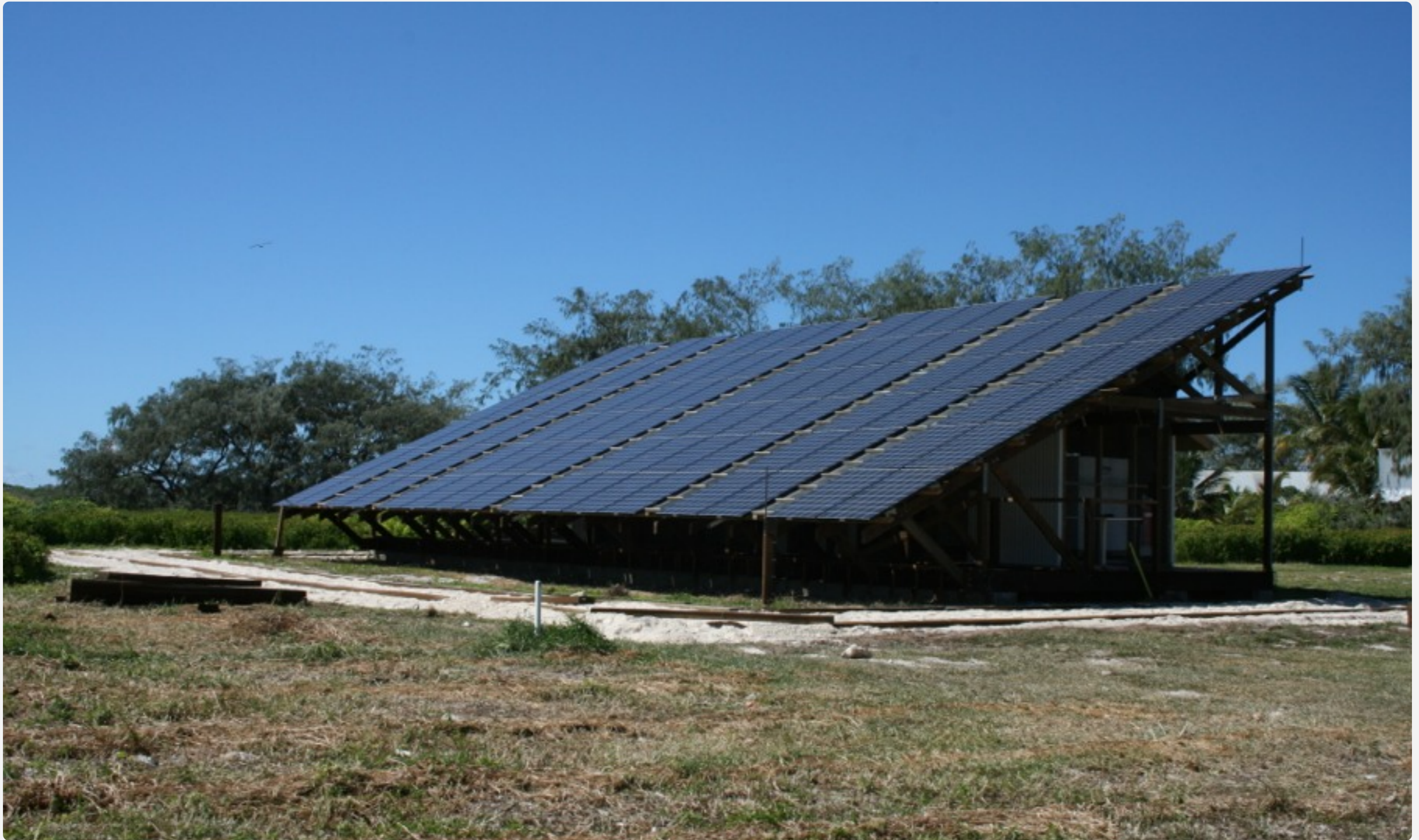
The solar array with power station beneath.
